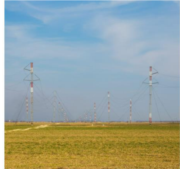
Emergency restoration of the overhead transmission lines with temporary towers, from 0.4 kV to 750 kV
