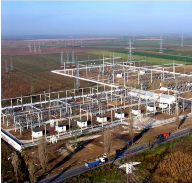
Power stations 750/400/20/110/20 kV and Substations 20/10/6/0.4 kV
