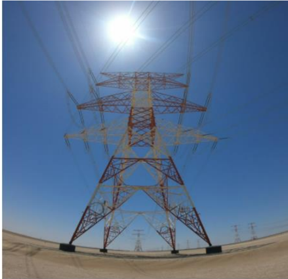
Overhead power lines from 0.4 kV to 750 kV
